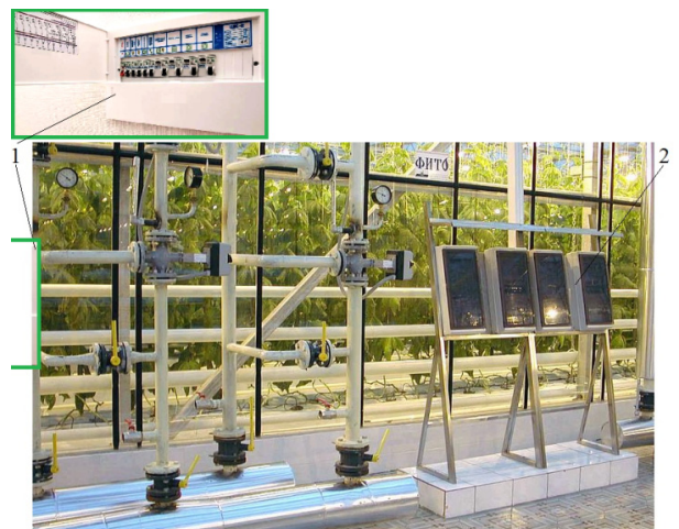
Fig. 3. Appearance of the climate control system. "1" indicates electric panel and "2" climate control system.
